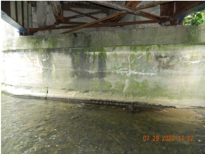
CRACKING AND SCALING IN WEST ABUTMENT
