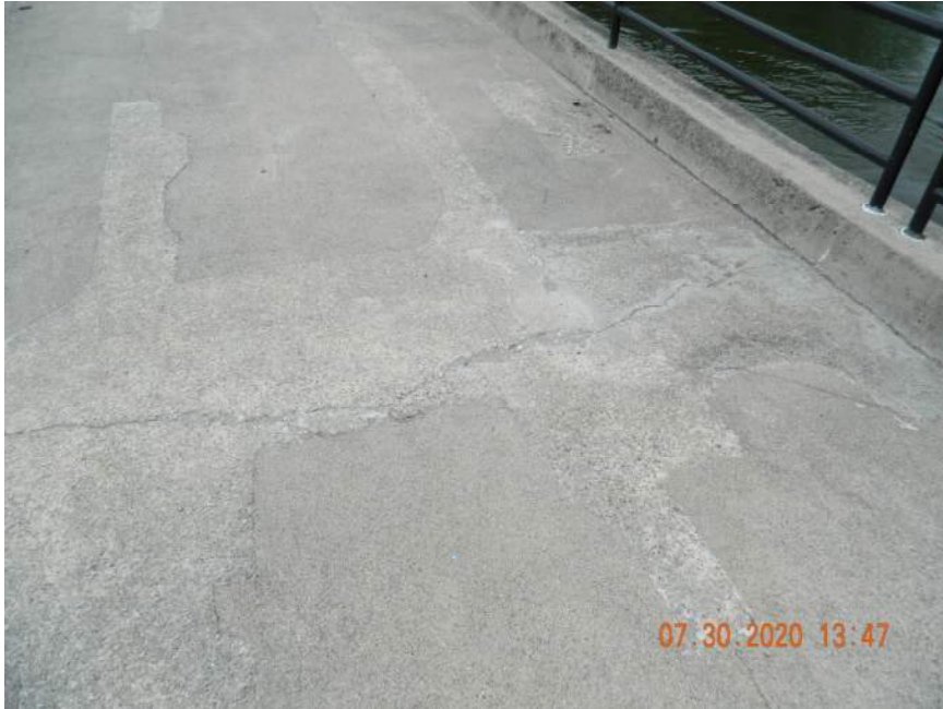
TYP. CRACKING IN DECK SURFACE
