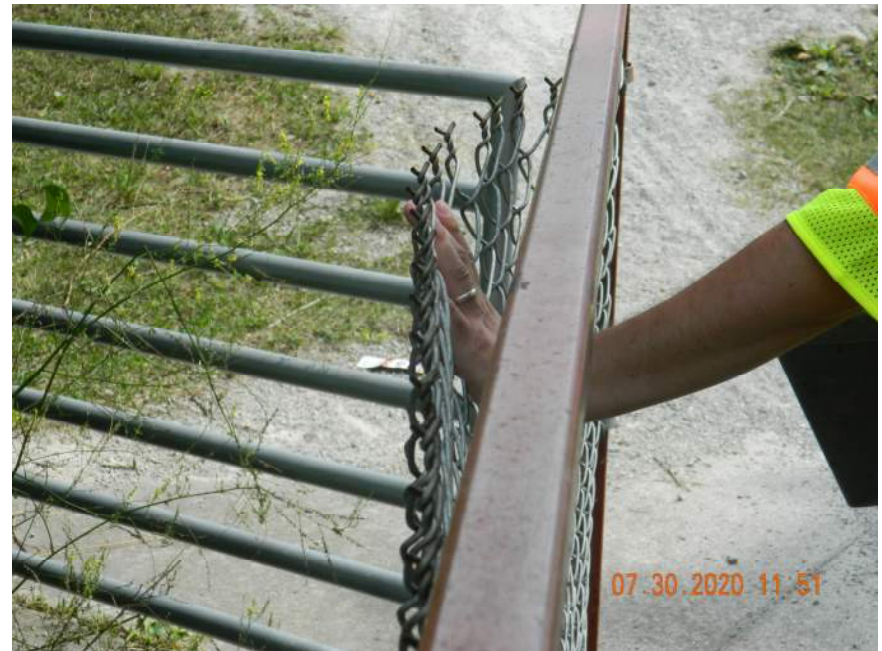
LOOSE FENCE IN NORTH RAIL AT EAST END
