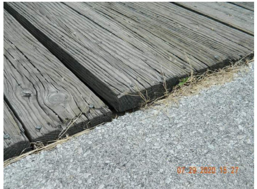
LOOSE TIMBER BOARDS AT WEST END
