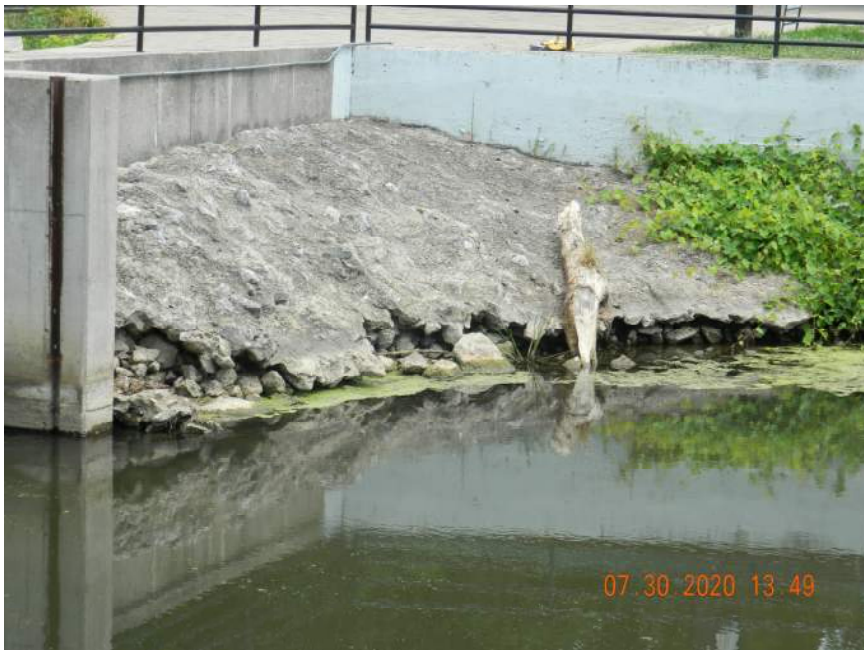
TYP. VOIDS IN GROUTED RIPRAP
