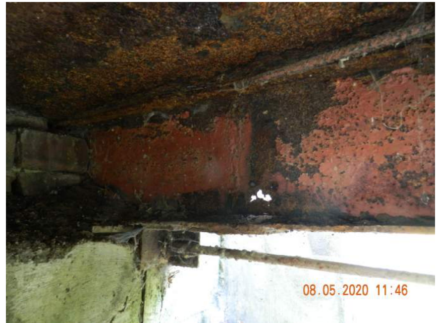
HOLE IN NORTH BEAM AT WEST BEARING
