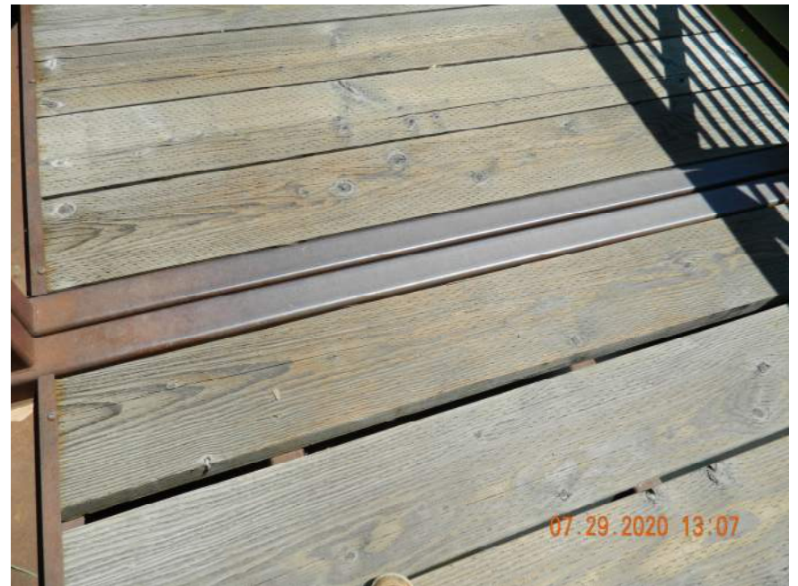
LOOSE DECK BOARD AT EAST PIER
