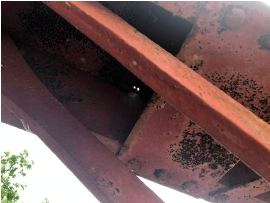
PITTING AND MINOR SECTION LOSS AT UPPER CHORD
