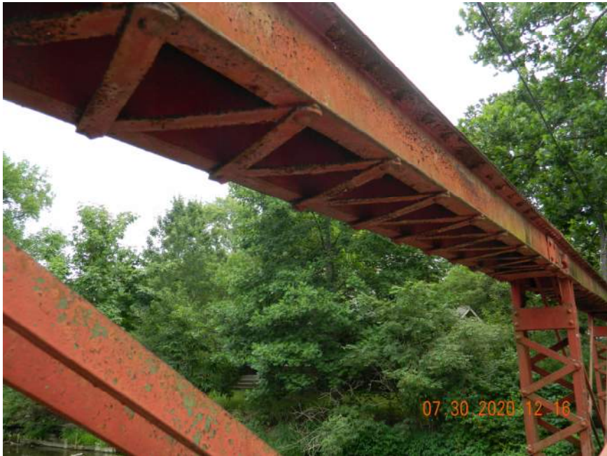
TYP. PITTING AND PAINT PEELING OF TRUSS
