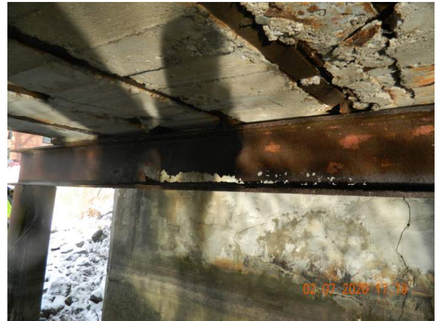
SECTION LOSS OF CAP BEAM AT BENT 6
