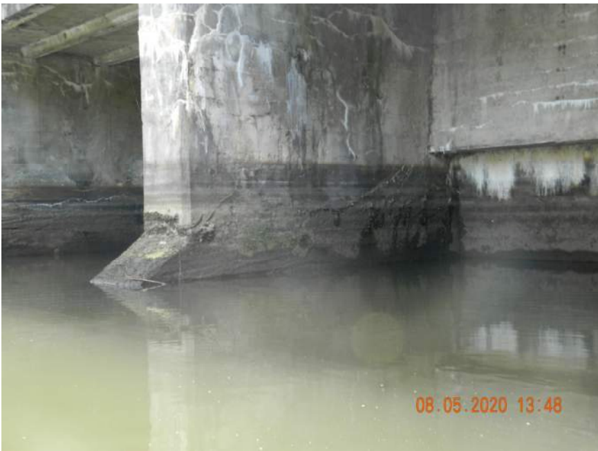
TYP. SCALING BELOW THE WATERLINE
