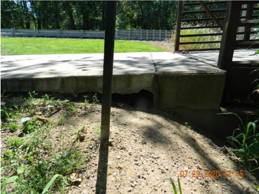
UNDERMINING AT EAST APPROACH
