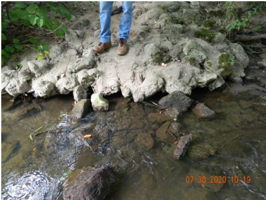
UNDERMINING AT TOE OF SOUTH SPILL SLOPE
