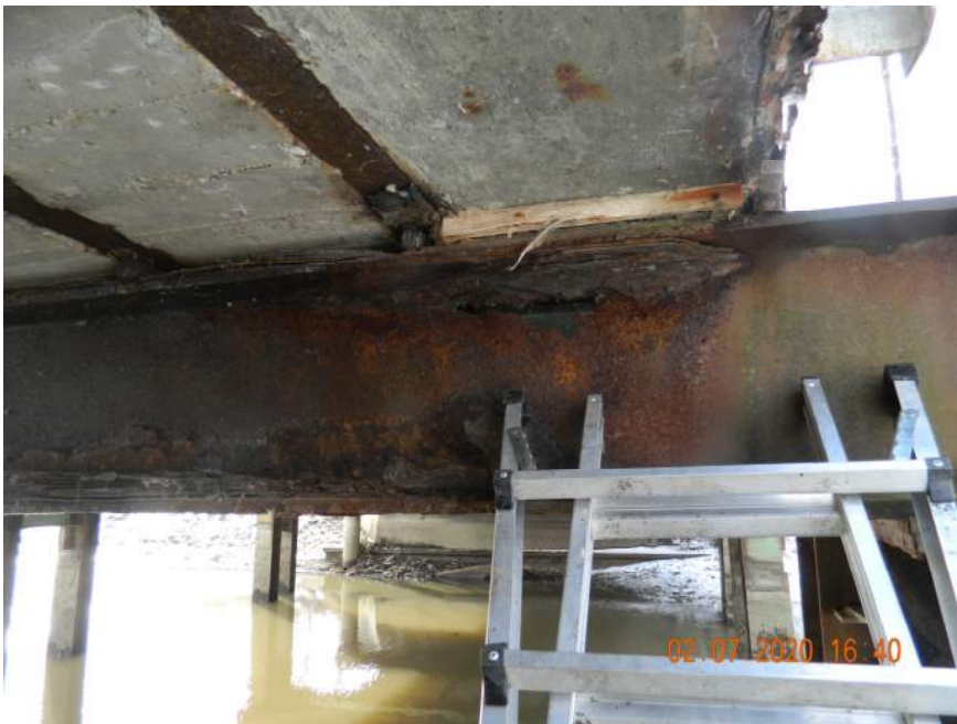
SECTION LOSS OF EAST BENT CAP BEAM AT BENT 5
