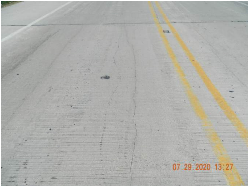
LONGITUDINAL CRACKING IN SLAB SURFACE
