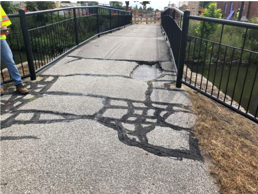
SETTLEMENT AND CRACKING OF WEST APPR. PAVMT.
