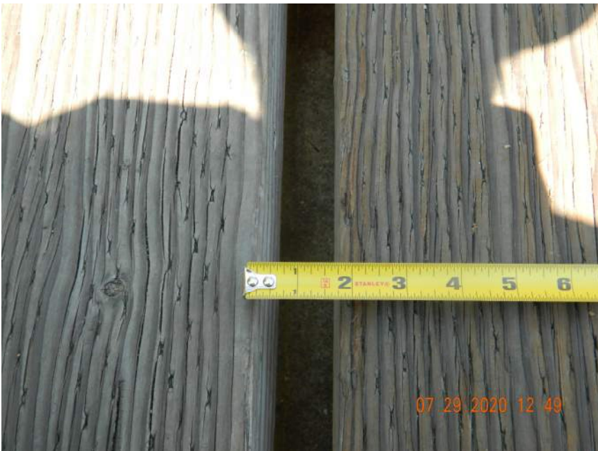
SEPARATION OF TIMBER BOARDS
