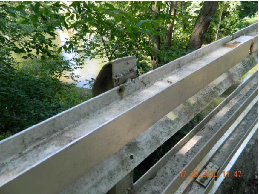
WELD FAILURE AT SOUTHEAST END OF RAIL
