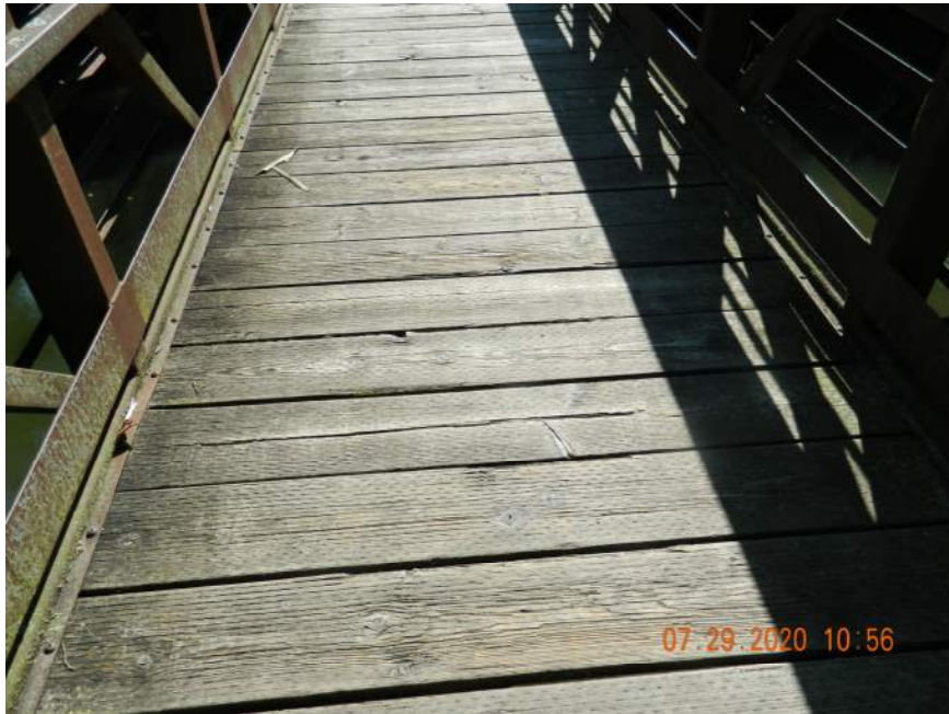
TYPICAL SPLITS & CHECKS IN TIMBER DECK
