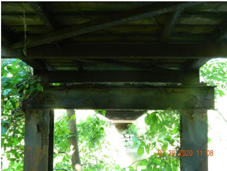
RUST AND PAINT PEELING IN CENTER PIER
