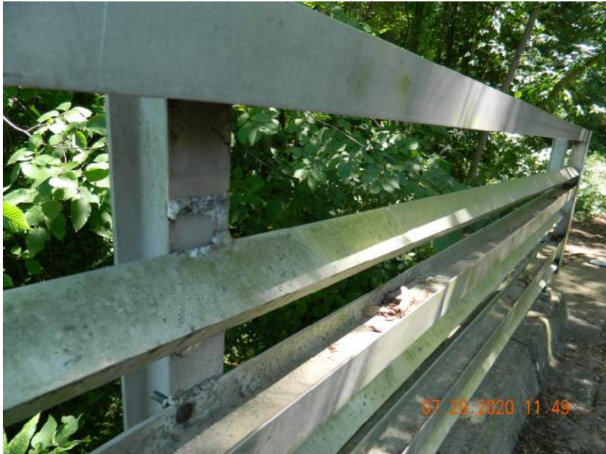
WELD FAILURE AT NORTHEAST END OF RAIL
