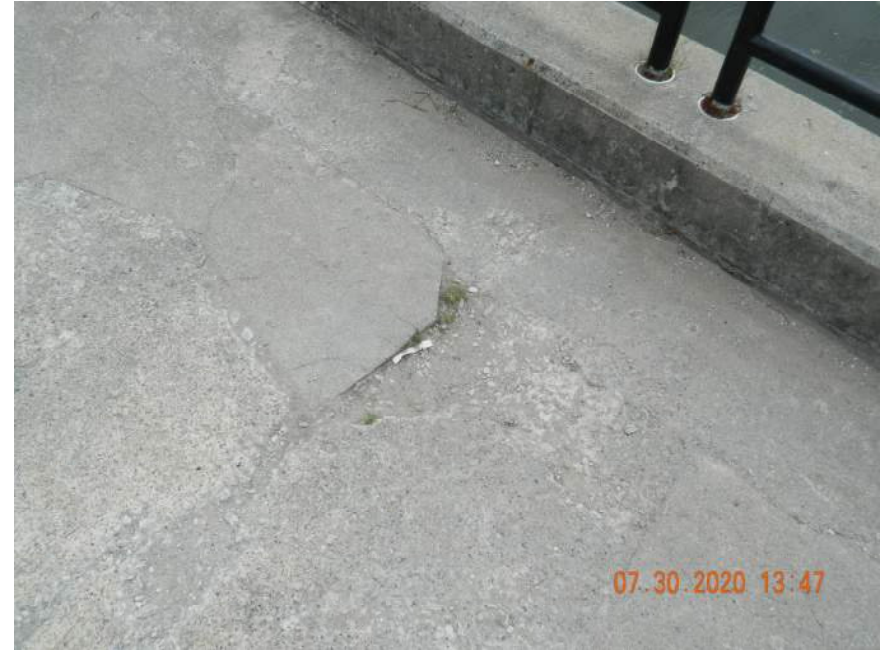
CRACKING AND SCALING IN DECK SURFACE
