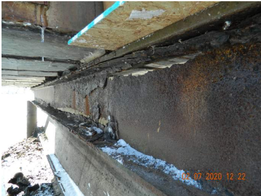
SECTION LOSS OF CAP BEAM AT BENT 2
