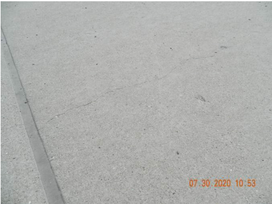
MINOR CRACKS IN SOUTH APPROACH SLAB
