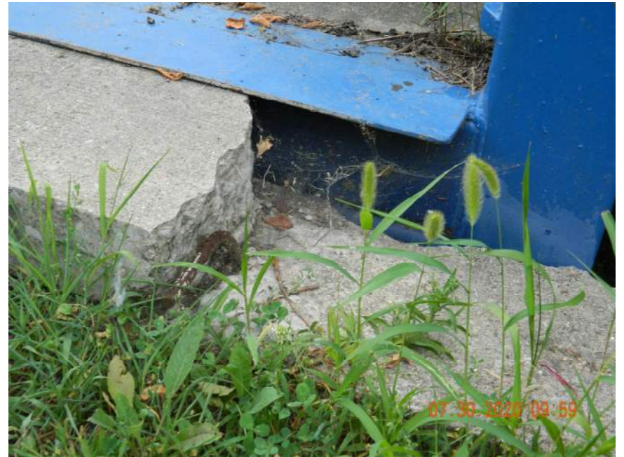
SPALL IN WEST CORNER OF NORTH END BENT MUDWALL
