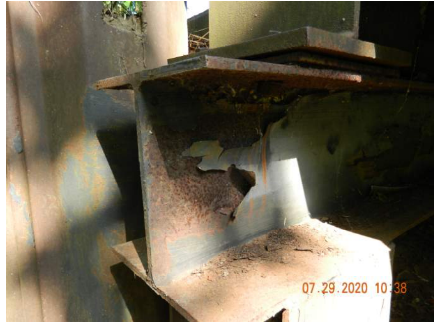
TYPICAL RUST AT END BENTS
