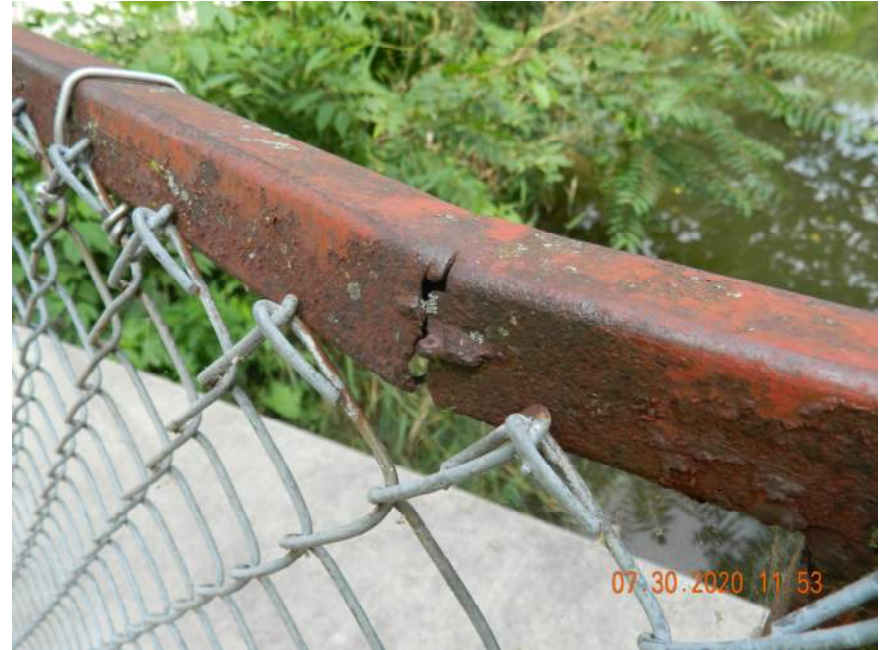
BROKEN TOP BAR IN BENT RAIL AT WEST END
