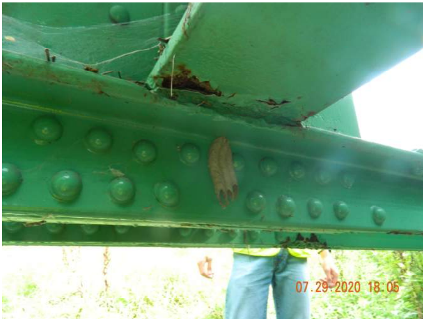
TYP. PACK RUST AT FLOORBEAM TO LOWER CHORD CONN.
