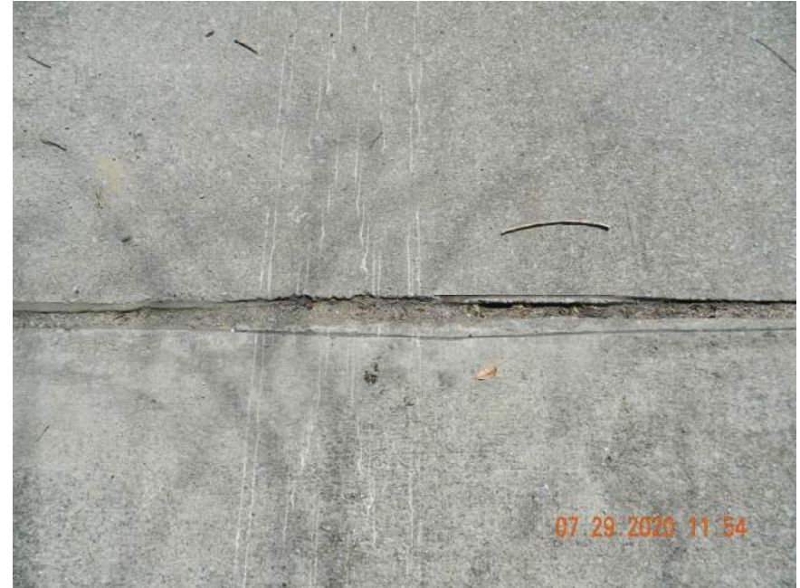
FAILED WEST EXPANSION JOINT DECK
