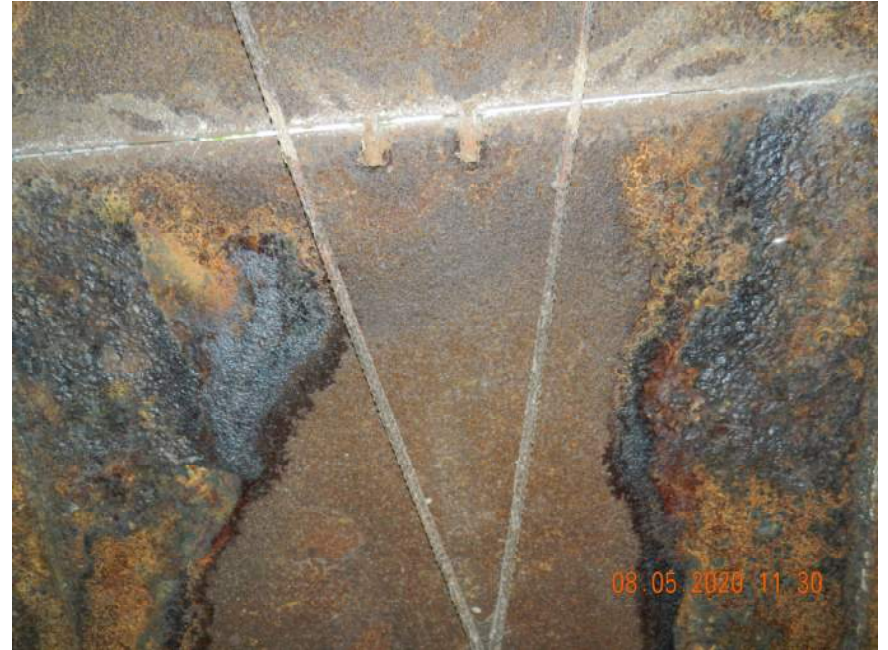
RUST AND SEPARATION OF DECK PL NEAR MIDSPAN
