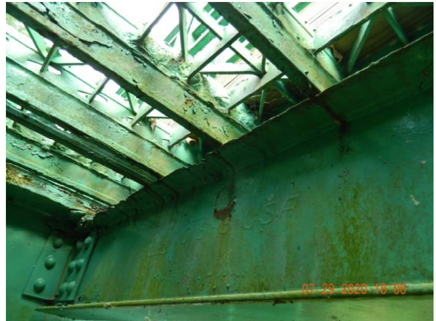
SECTION LOSS IN TOP FLANGE OF STRINGERS
