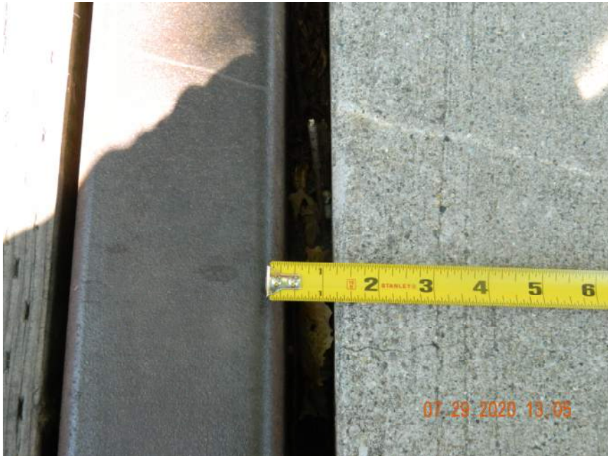
>1" SEPARATION AT EAST APPROACH END
