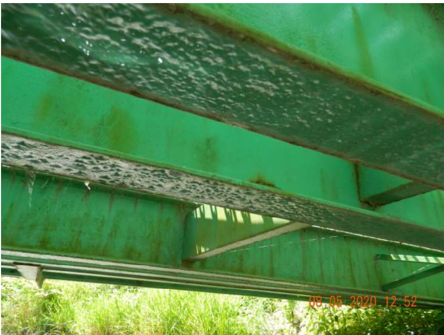
TYPICAL PITTING OF STEEL BEAMS
