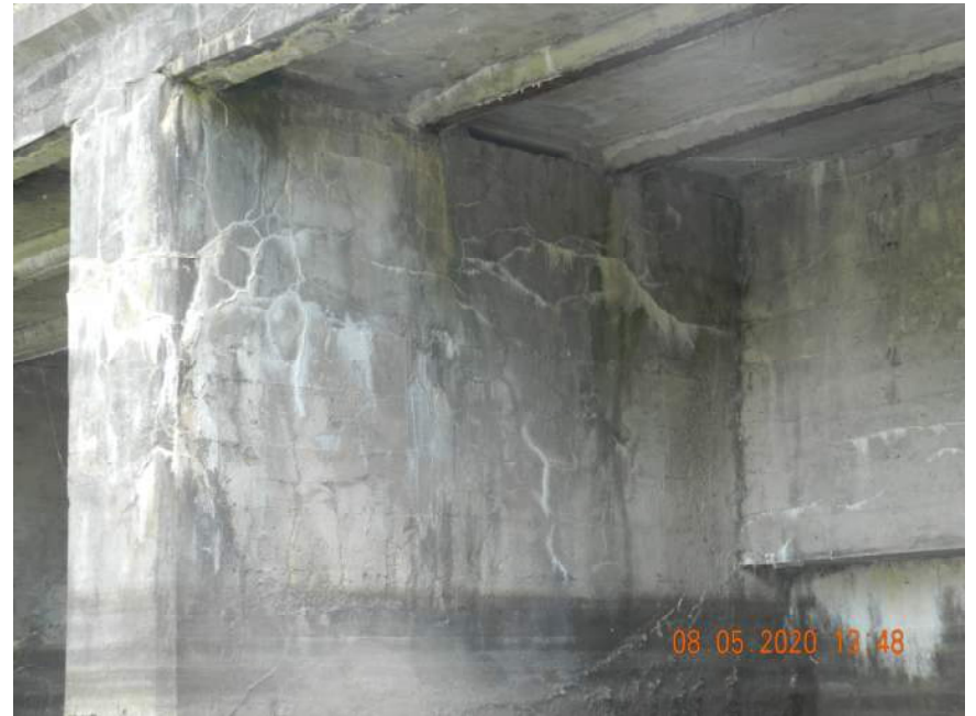
HEAVY CRACKING WITH LEACHING IN WEST PIER
