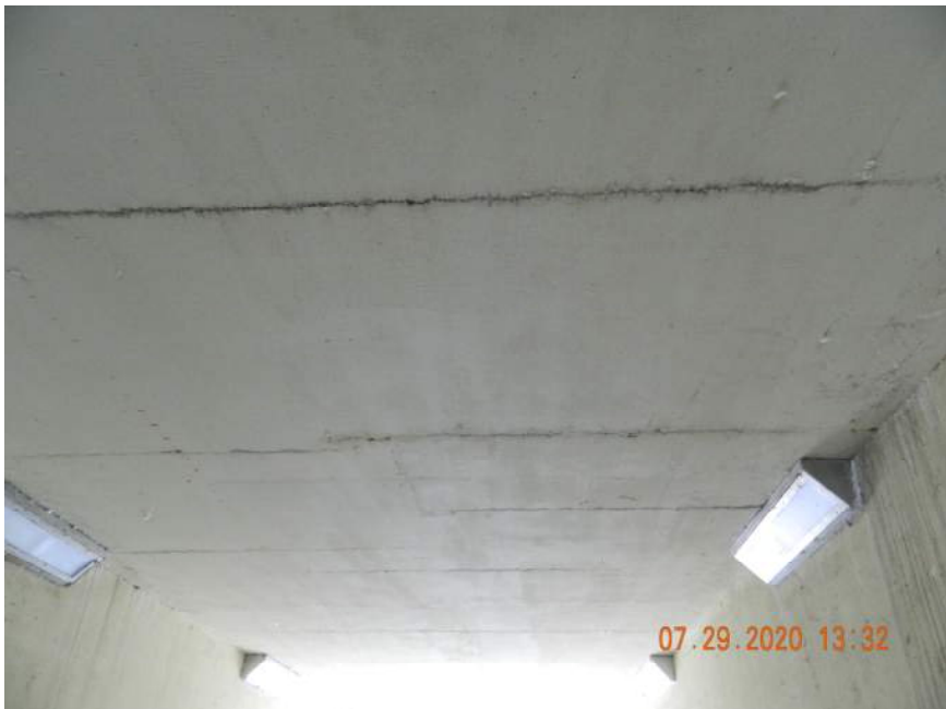
LONGITUDINAL CRACKING IN UNDERSIDE OF TOP SLAB
