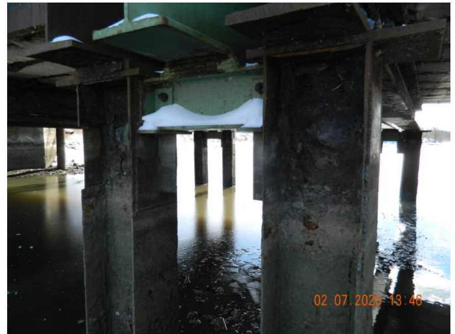
TYPICAL HEAVY RUST OF H-PILES
