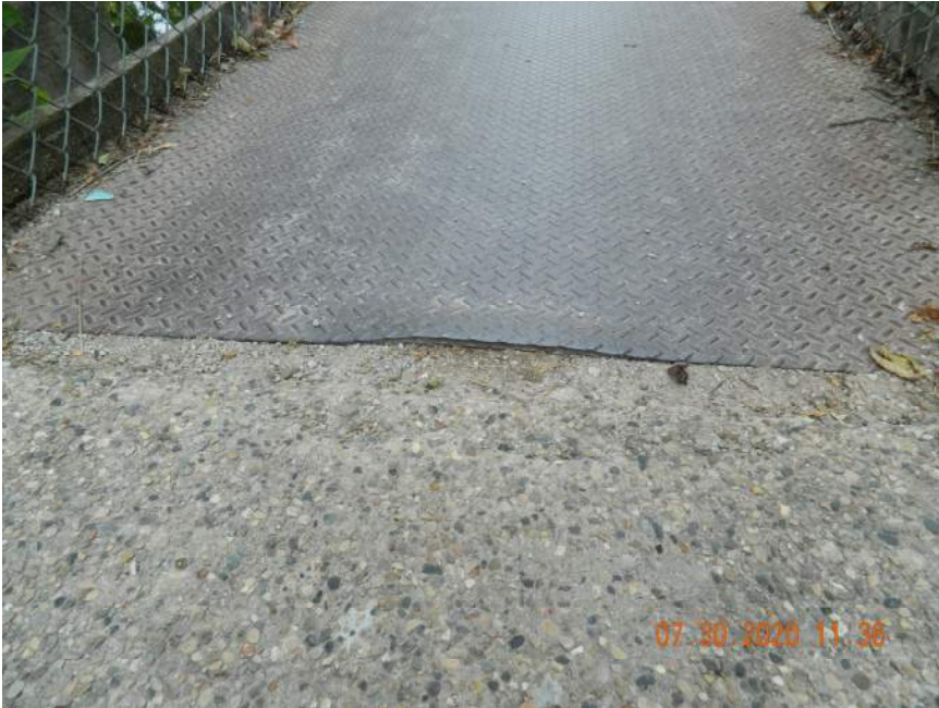
DENT IN DECK PLATE AT EAST END
