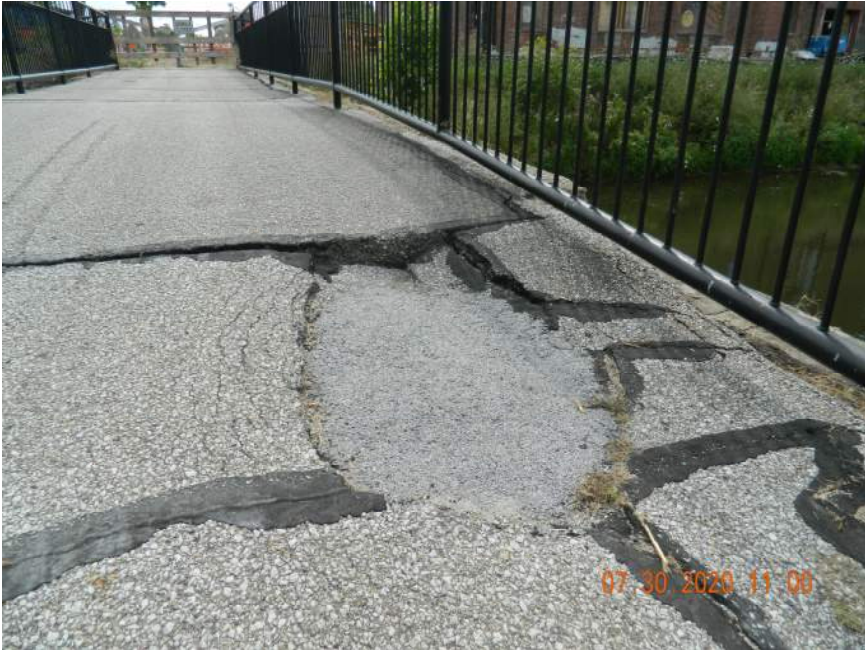
SETTLEMENT IN WEST APPROACH
