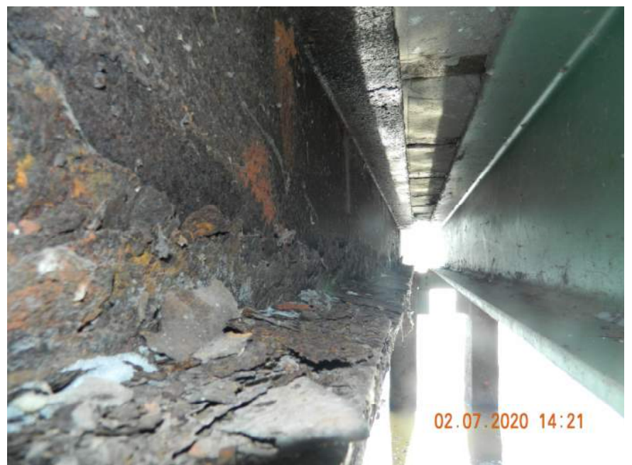
TYP. PACK RUST IN ORIGINAL BENT CAPS AT BENTS 3, 4 & 5
