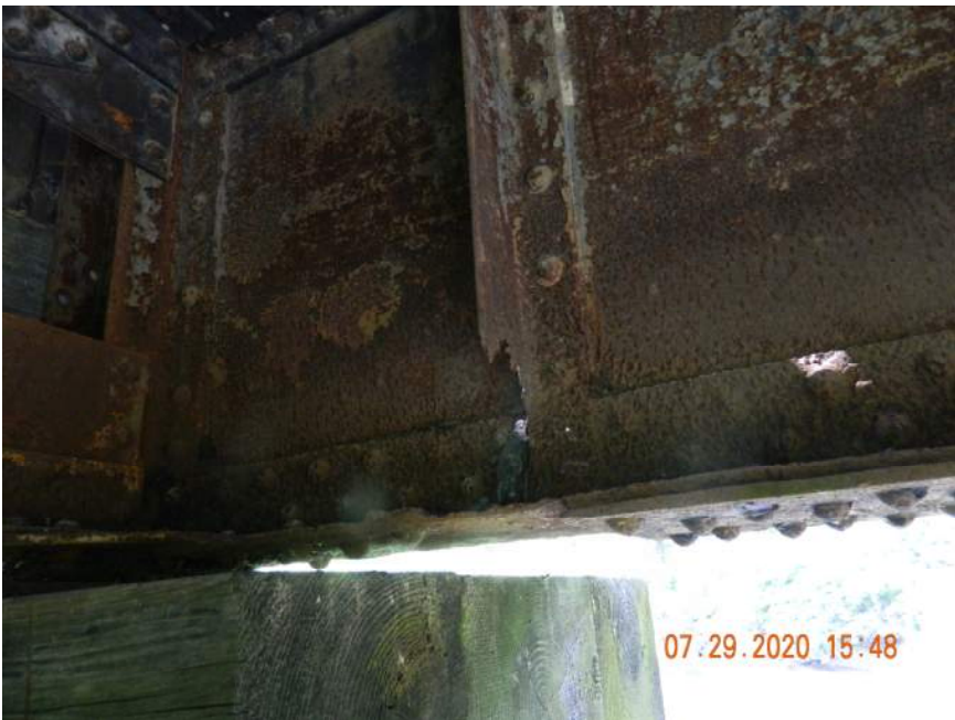
100% SECTION LOSS IN STEEL STIFFENERS
