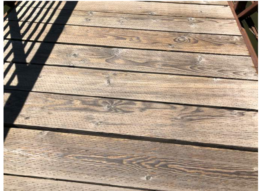
SEPARATION OF TIMBER BOARDS
