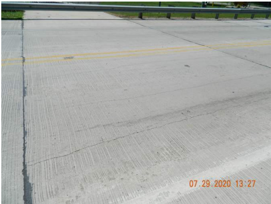
LONGITUDINAL CRACKING IN SLAB SURFACE
