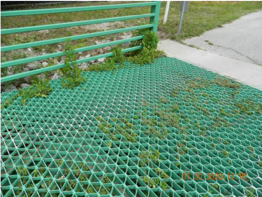
VEGETATION GROWING UNDER EAST END OF BRIDGE
