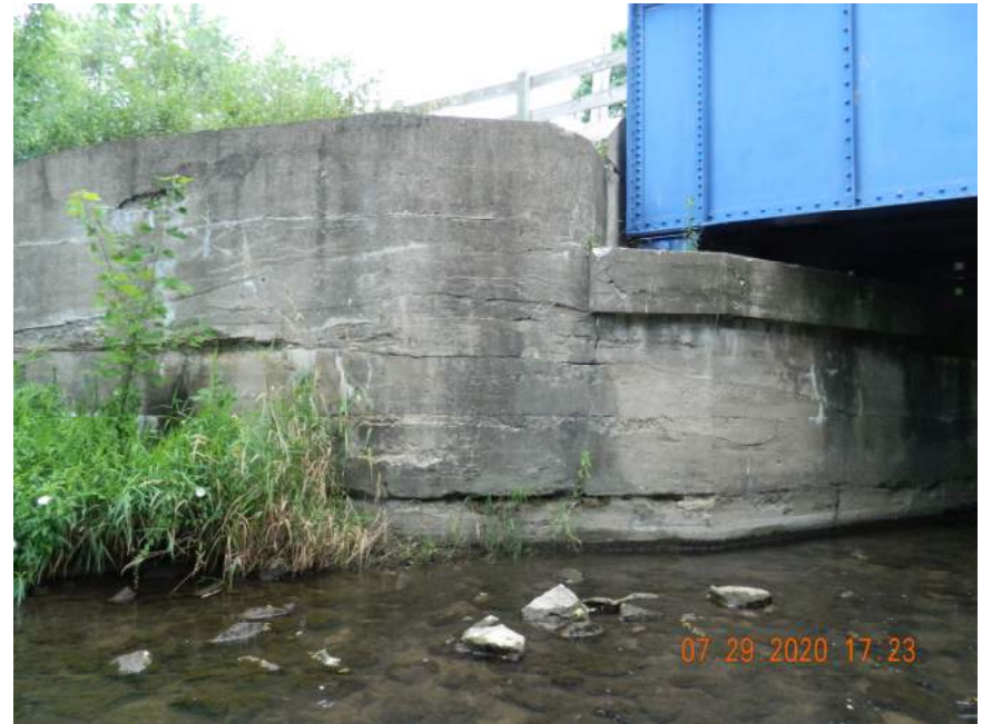
SCALING AND ABRASION IN EAST ABUTMENT
