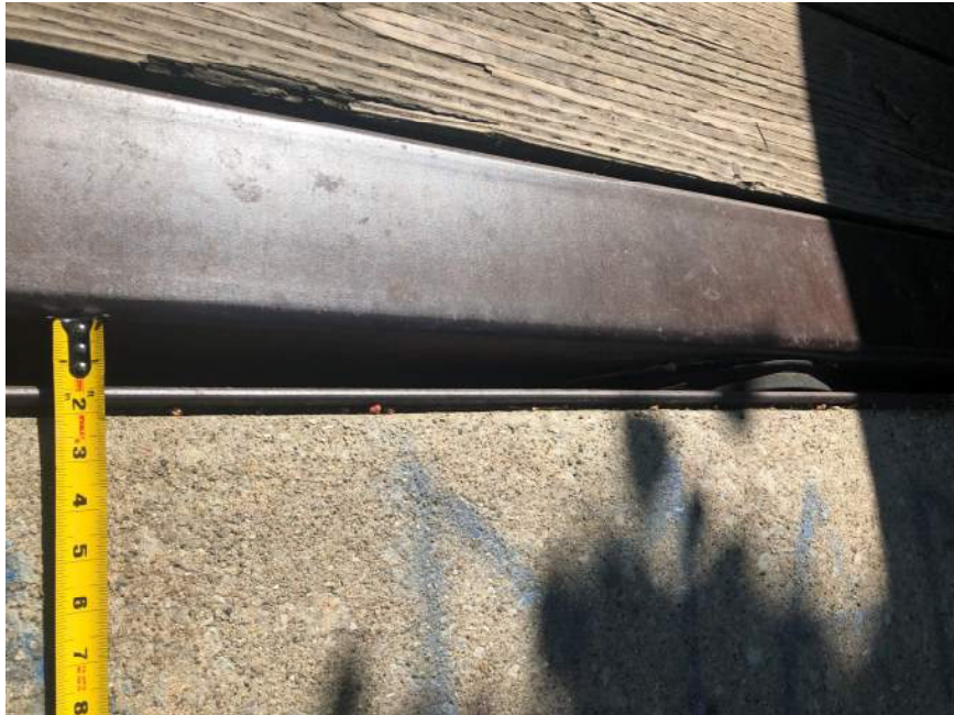
EXPANSION JOINT AT WEST END MISSING MATERIAL
