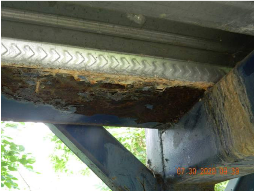
TYP. LEACHING AND RUST AT TRUSS/ DECK INTERFACE
