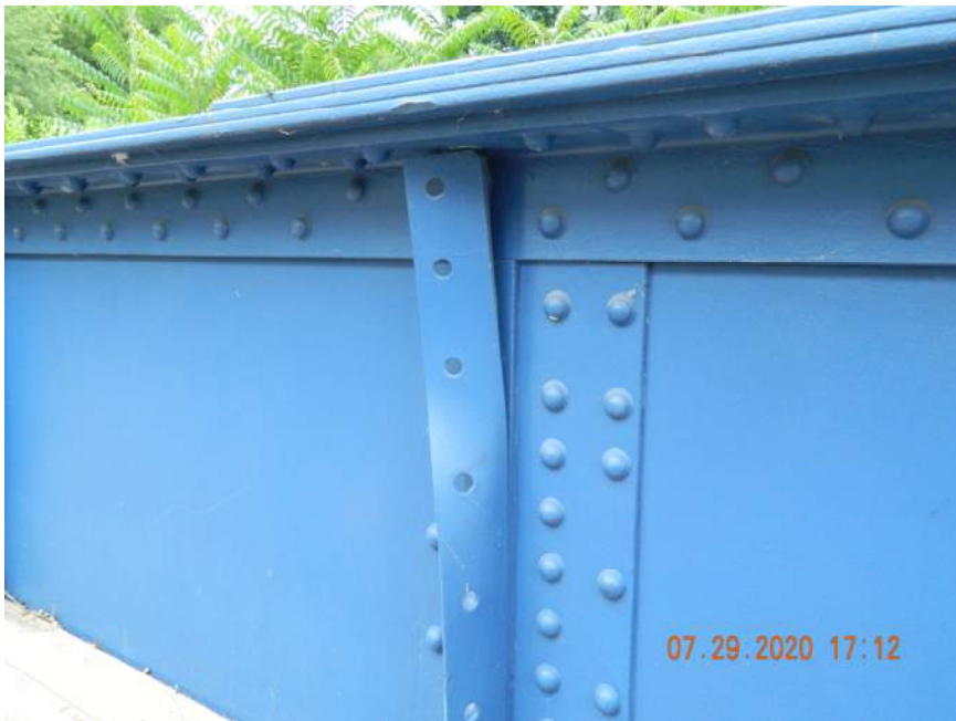
TWISTED STEEL STIFFENER ABOVE DECK
