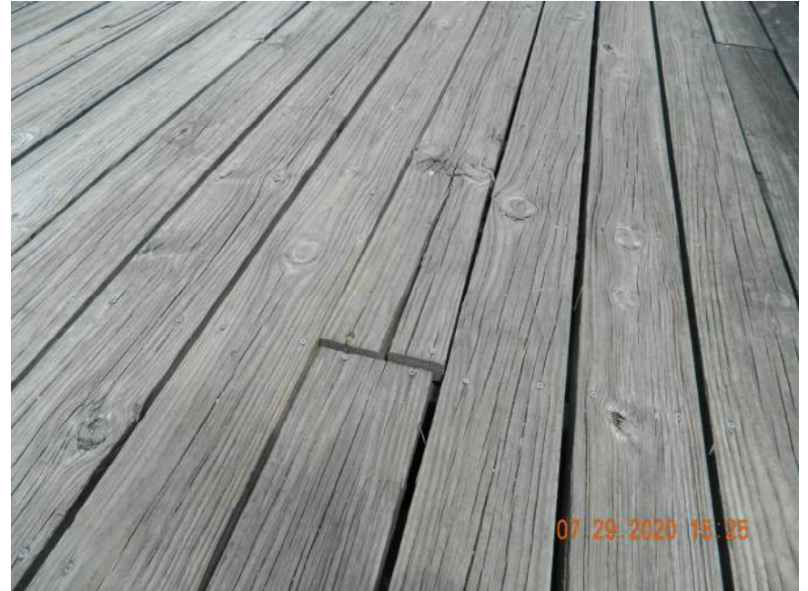
SPLITTING OF TIMBER DECK BOARDS
