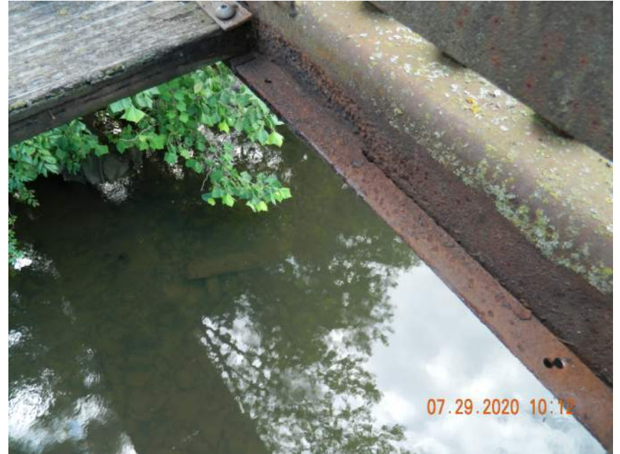
RUST AND PITTING AT LOWER CHORDS NEXT TO BOARDS
