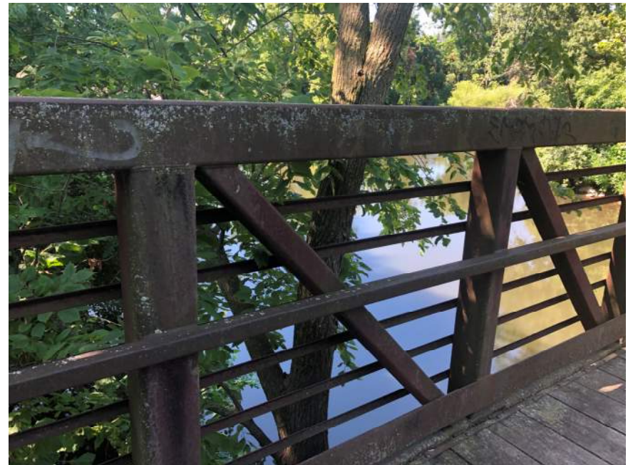
TREE NEXT TO SOUTH TRUSS KEEPING BRIDGE WET
