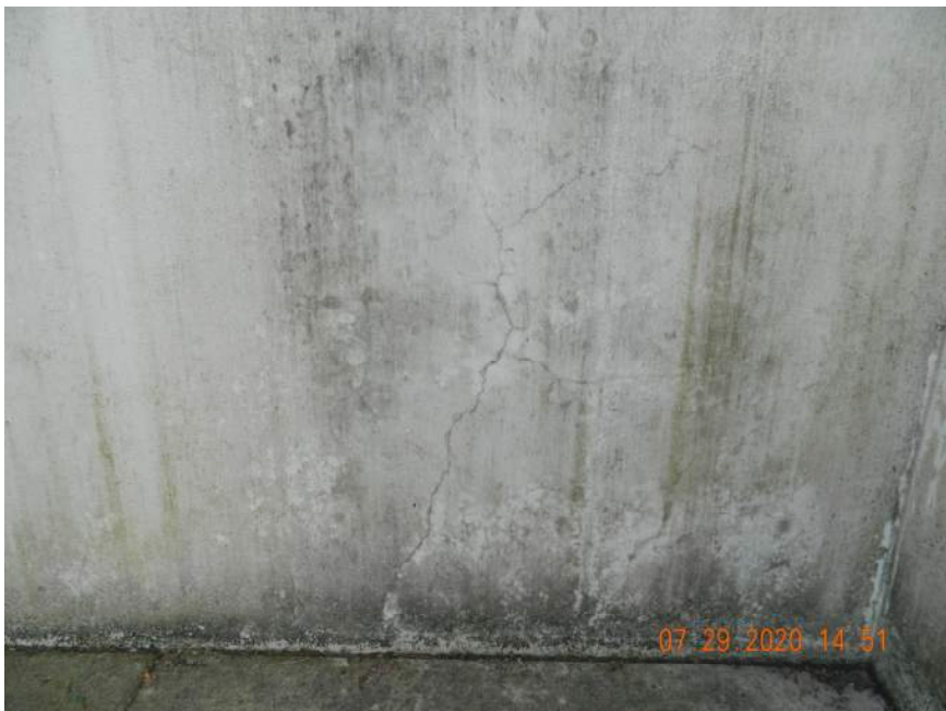
MINOR SHRINKAGE CRACKS IN WEST STAIRS RET. WALL
