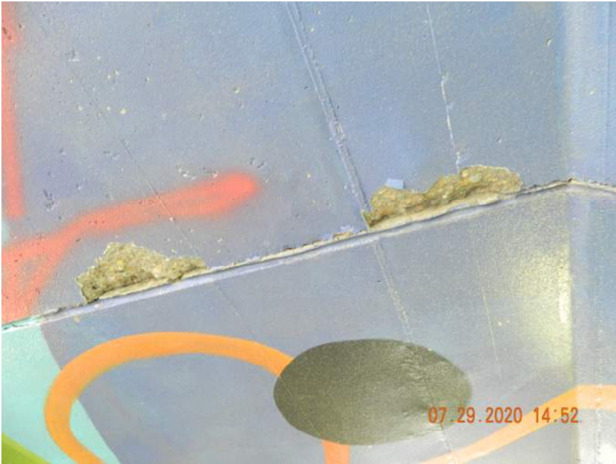
SURFACE SPALLS IN TOP SLAB OF UNIT 2 FROM WEST
