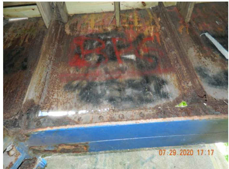
100% SECTION LOSS IN WEB PL OF S. GIRDER AT E. BRG.
