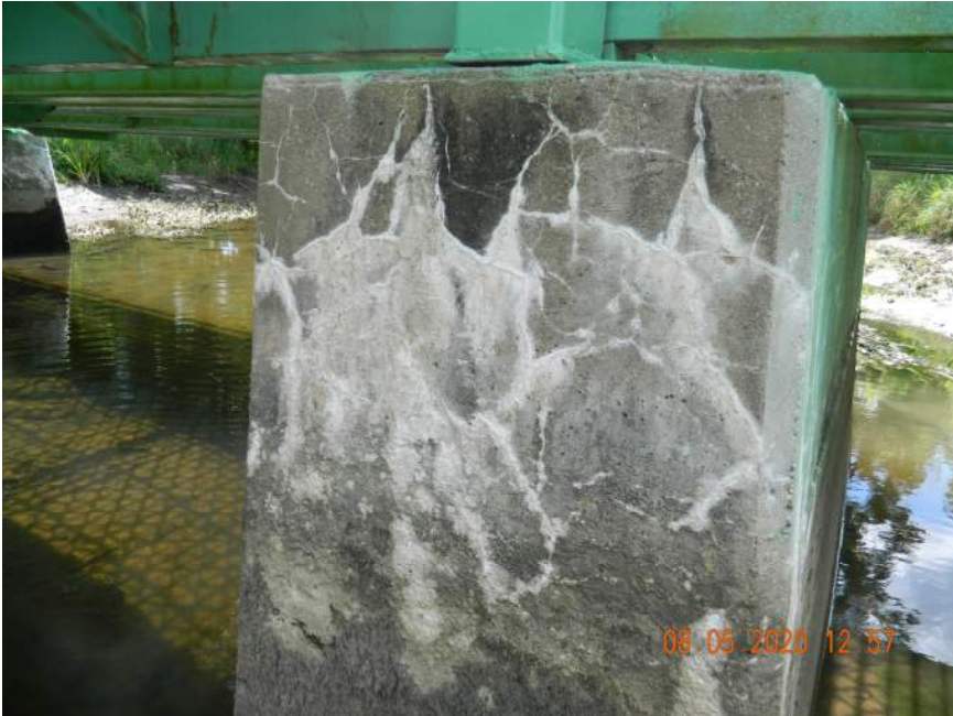
TYPICAL CRACKING WITH LEACHING AT PIERS
