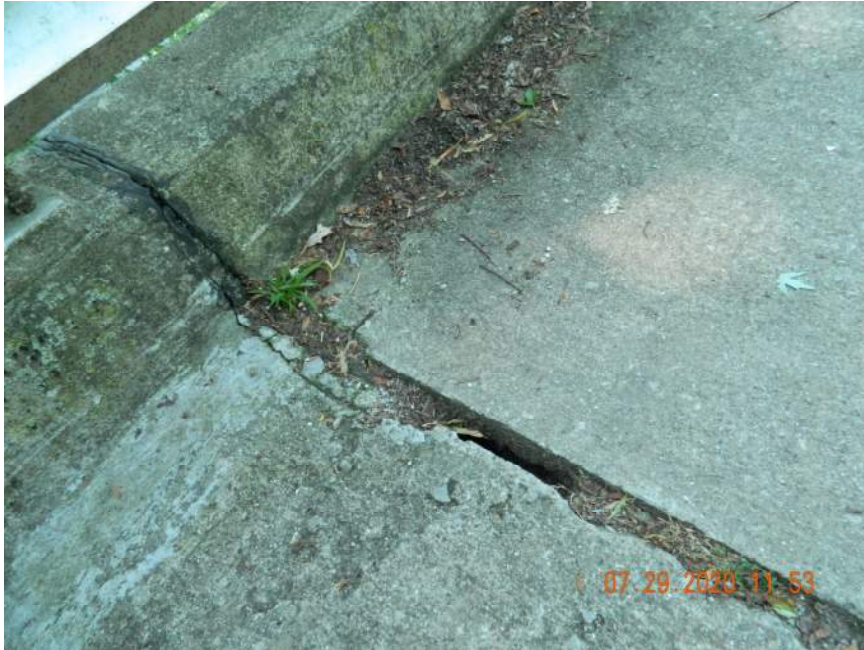
FAILED EAST EXPANSION JOINT DECK
