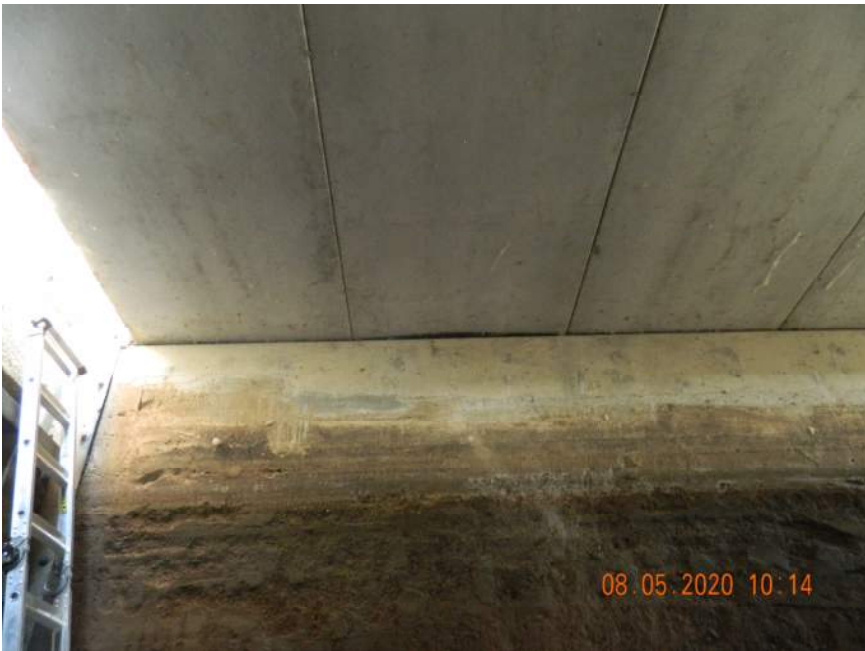
BEARING PAD EXPOSED IN BEAM 2 FROM W., S. SPAN
