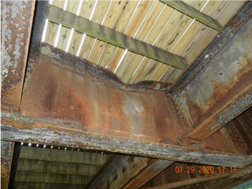
TYP. TWISTING IN TOP FLANGE AND WEB OF FLOORBEAMS
