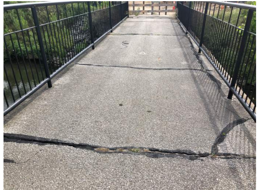
CRACKING OF PAVEMENT AT BRIDGE
