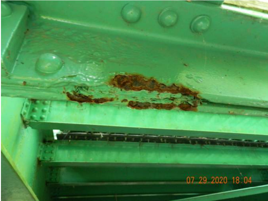
TYP. PACK RUST AT LOWER CHORD OF TRUSS
