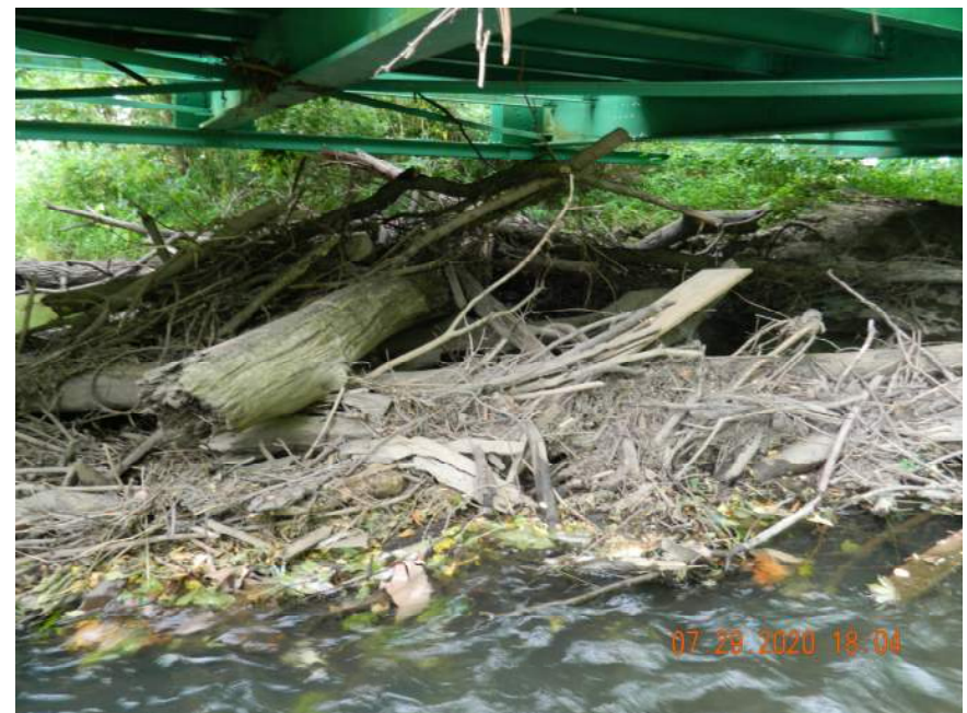
HEAVY DEBRIS IN CHANNEL
