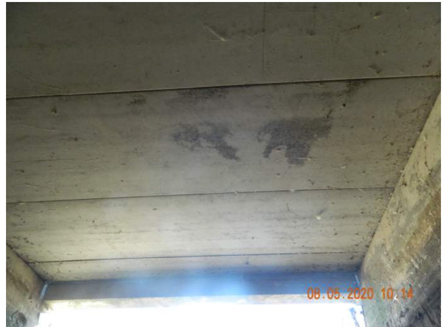
HONEYCOMB IN BEAM 4 FROM W., S. SPAN
