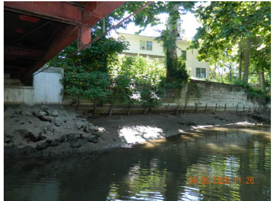
SOUTHEAST RETAINING WALL LEANING
