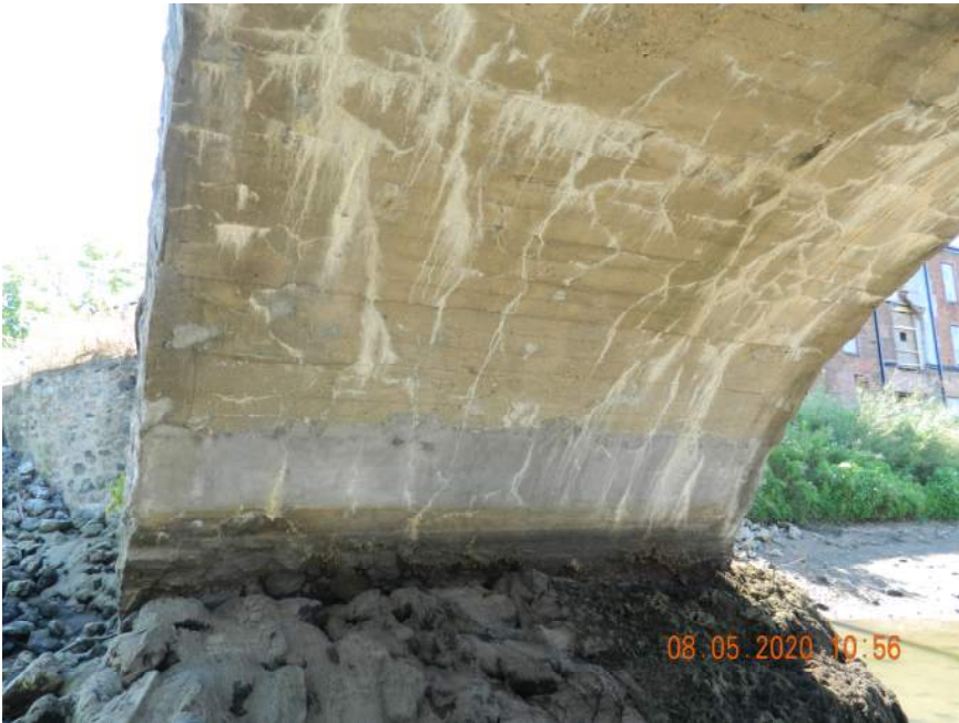
CRACKS WITH EFFLORESCE IN WEST SPAN AT PIER
