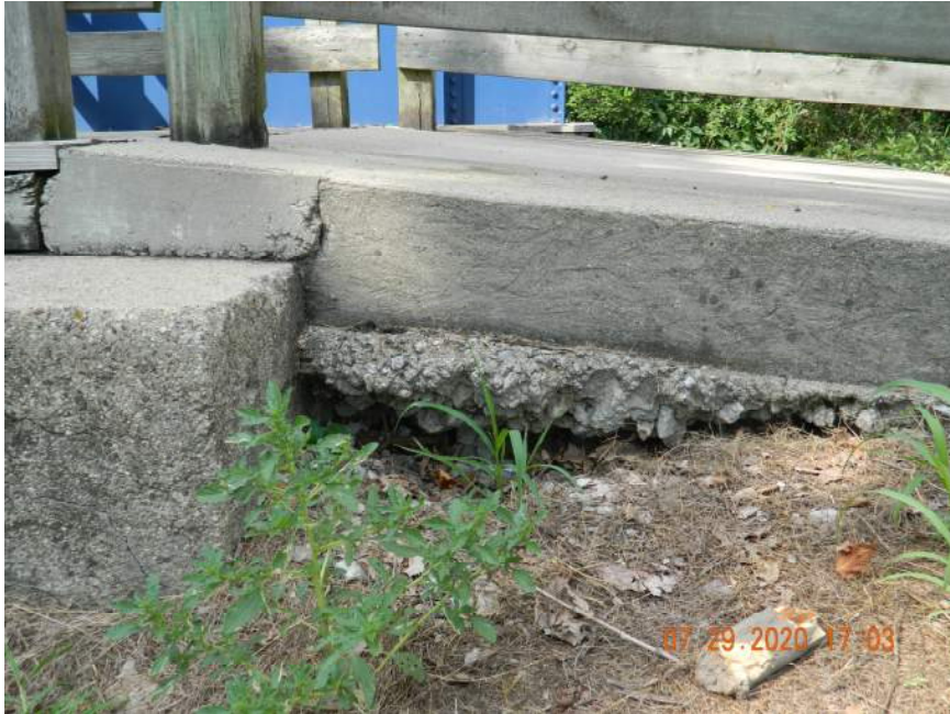
UNDERMINING IN EAST APPROACH
