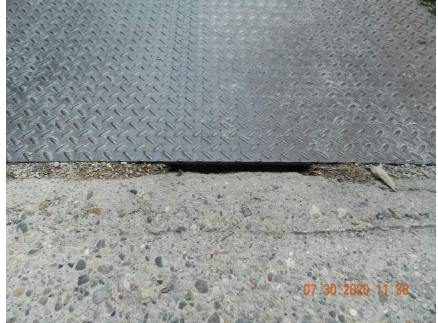
GAP AT WEST APPROACH END OF BRIDGE
