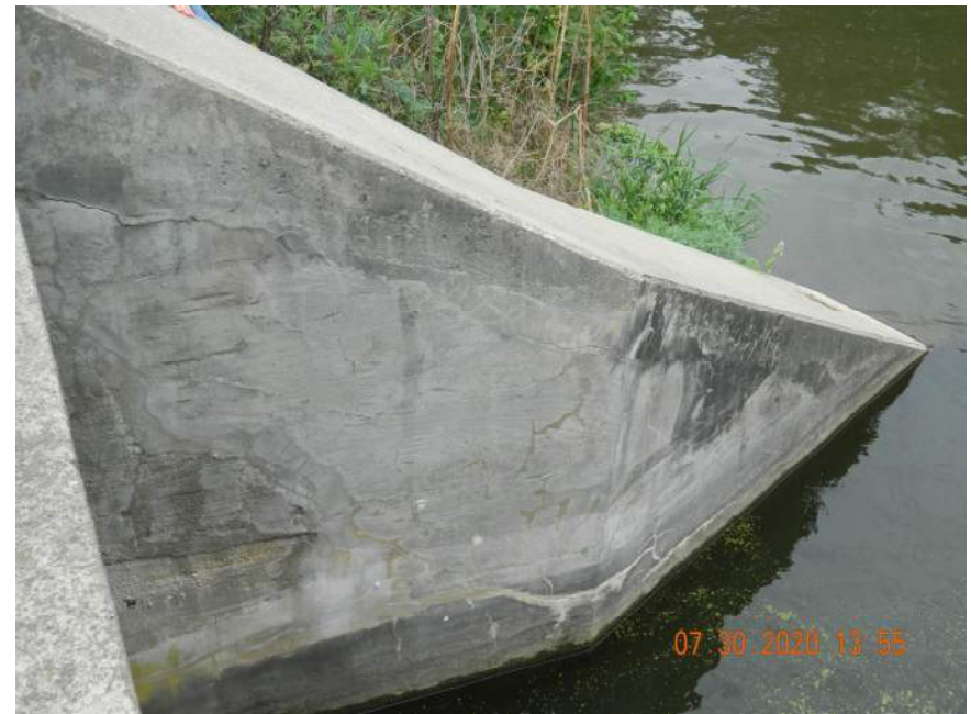
CRACKING IN NORTH WINGWALL OF WEST ABUTMENT
