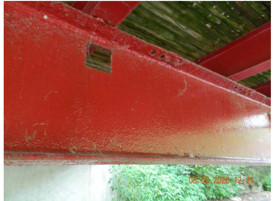
TYP. PITTING OF FLOORBEAMS
