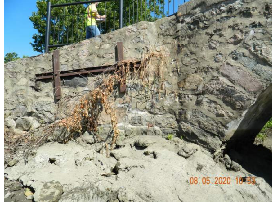
VOIDS AT SOUTHWEST WINGWALL
