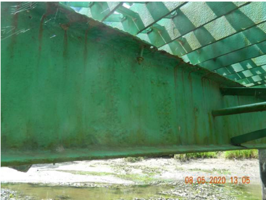
TYP. PITTING & SECTION LOSS ON FLANGES OF BEAMS
