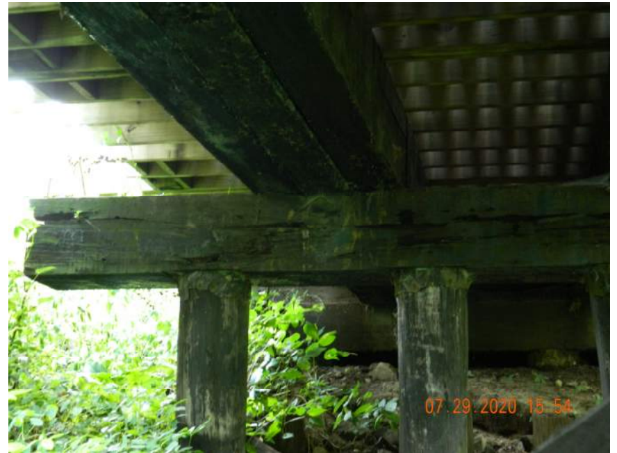
TYPICAL SPLITS IN PIER CAPS OF APPROACH SPANS
