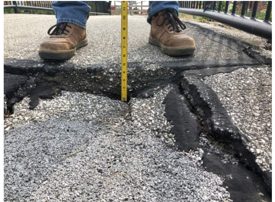
SETTLEMENT IN WEST APPROACH
