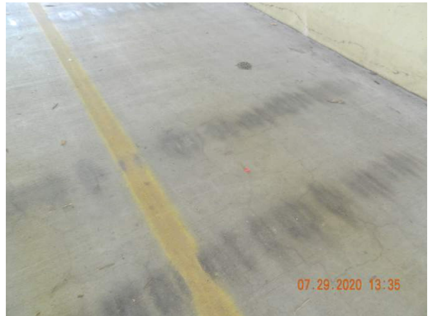
MINOR MAP CRACKING IN SURFACE OF BOTT. SLAB
