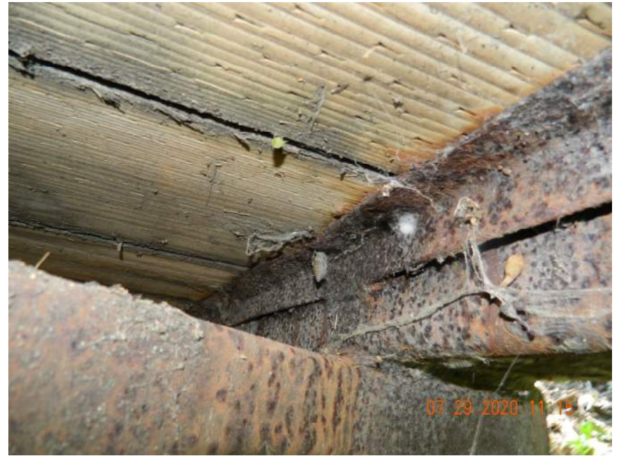
RUST AND PITTING BELOW TIMBER DECK
