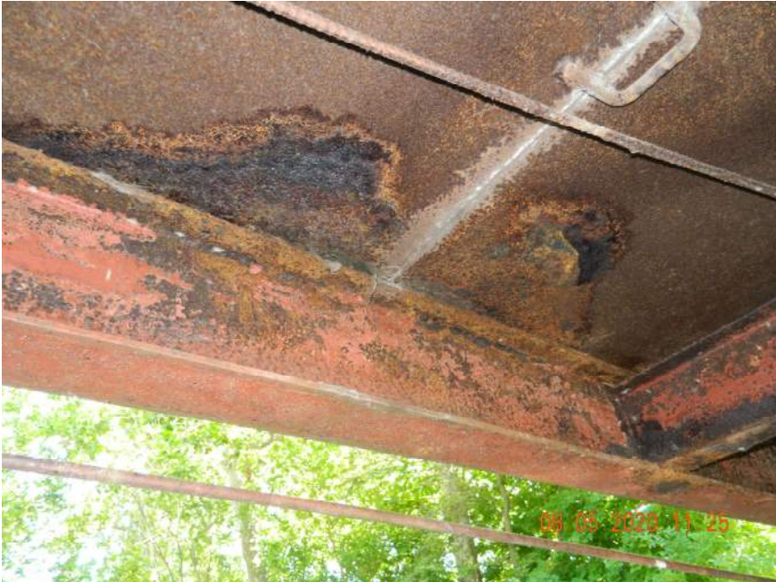
TYPICAL RUST & PITTING OF STEEL BEAMS AND DECK PL
