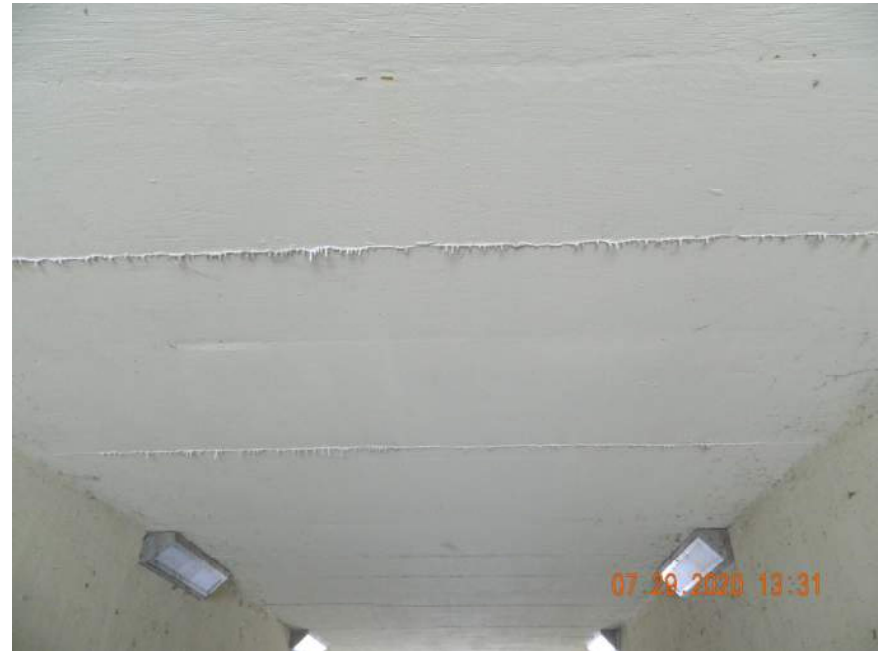
UNDERSIDE OF TOP SLAB W/ LONGITUDINAL CRACKING
