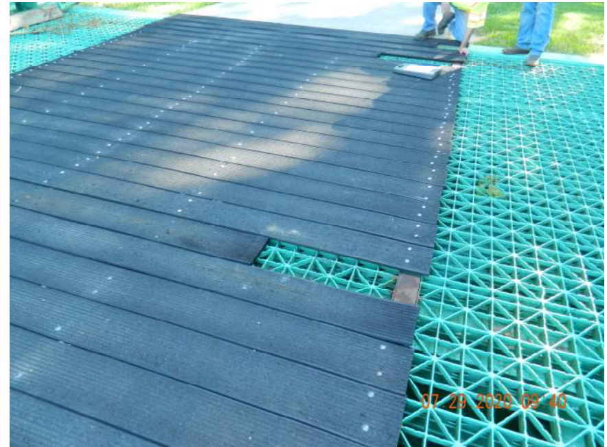
TYP. RUBBER MAT PIECES MISSING
