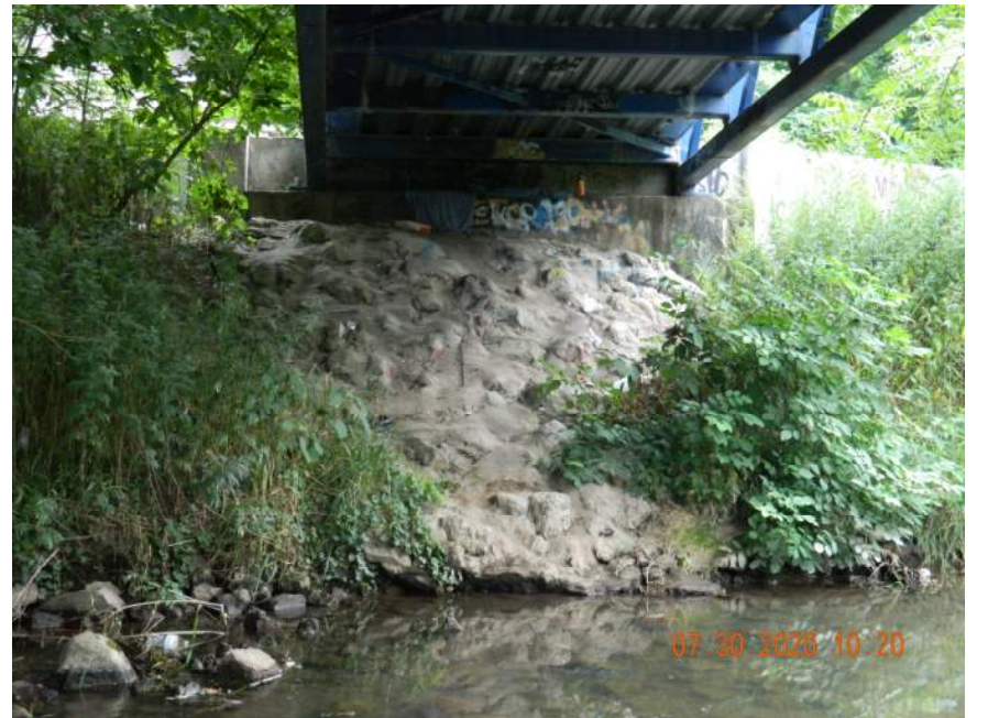
UNDERMINING AT TOE OF NORTH SPILL SLOPE
