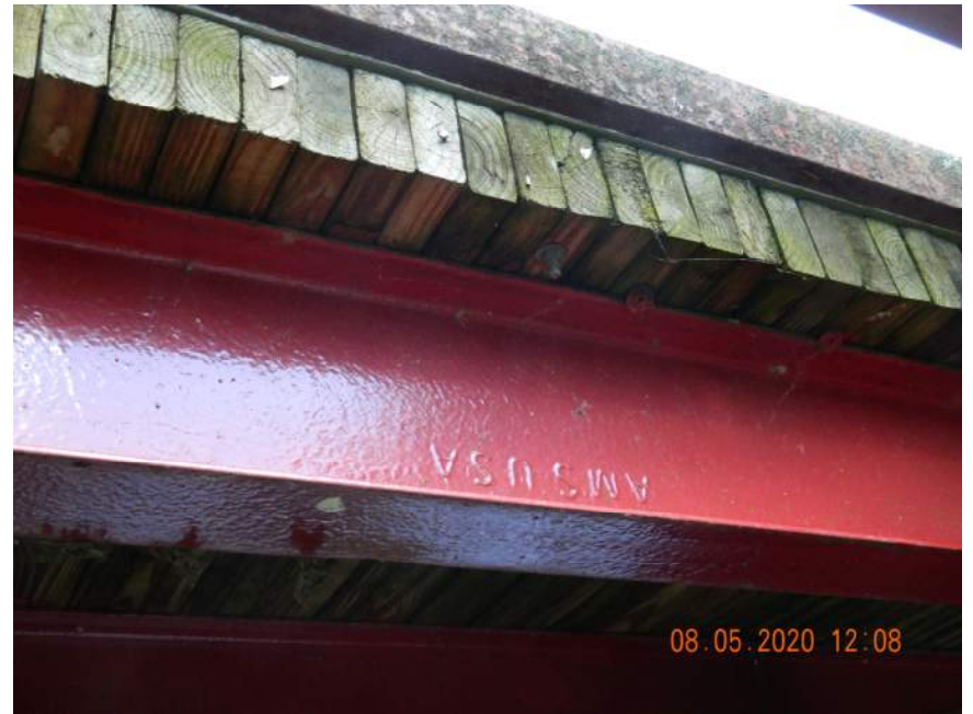
TYP. PITTING OF STRINGERS
