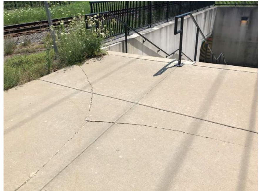
CRACKING IN SIDEWALK APPROACH AT WEST STAIRS
