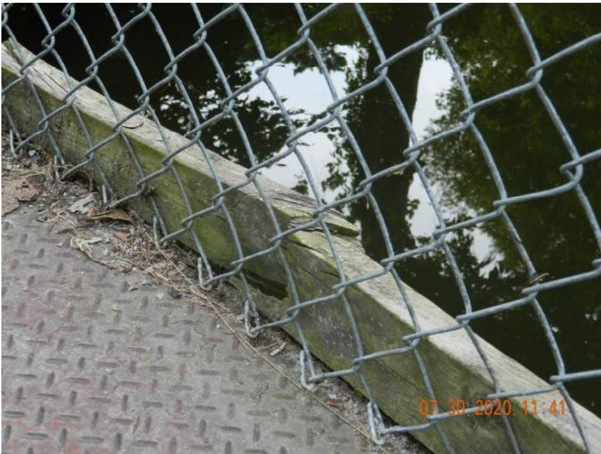
DAMAGED KICKBOARD IN SOUTH RAIL NEAR MIDSPAN
