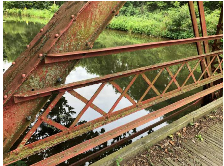
MOISTURE AND RUST IN SOUTH TRUSS AT EAST END
