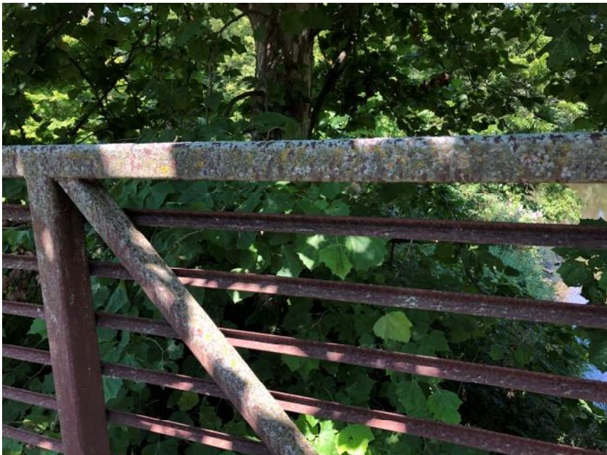
HEAVY VEGETATION NEXT TO NORTH TRUSS
