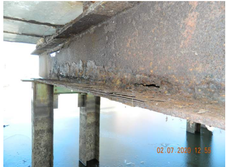
SECTION LOSS OF WEST BENT CAP BEAM AT BENT 3
