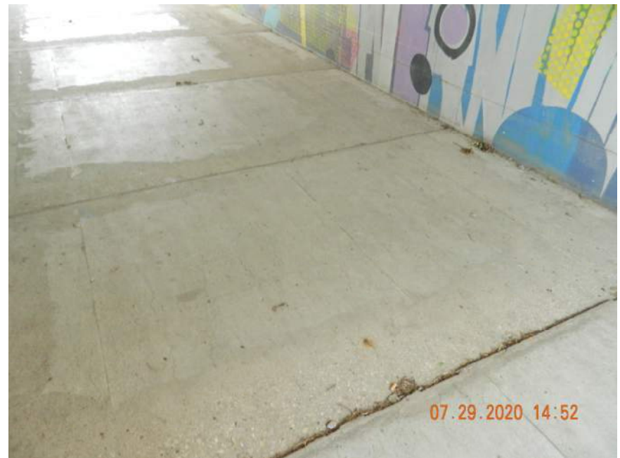
MINOR MAP CRACKING IN BOTTOM SLAB
