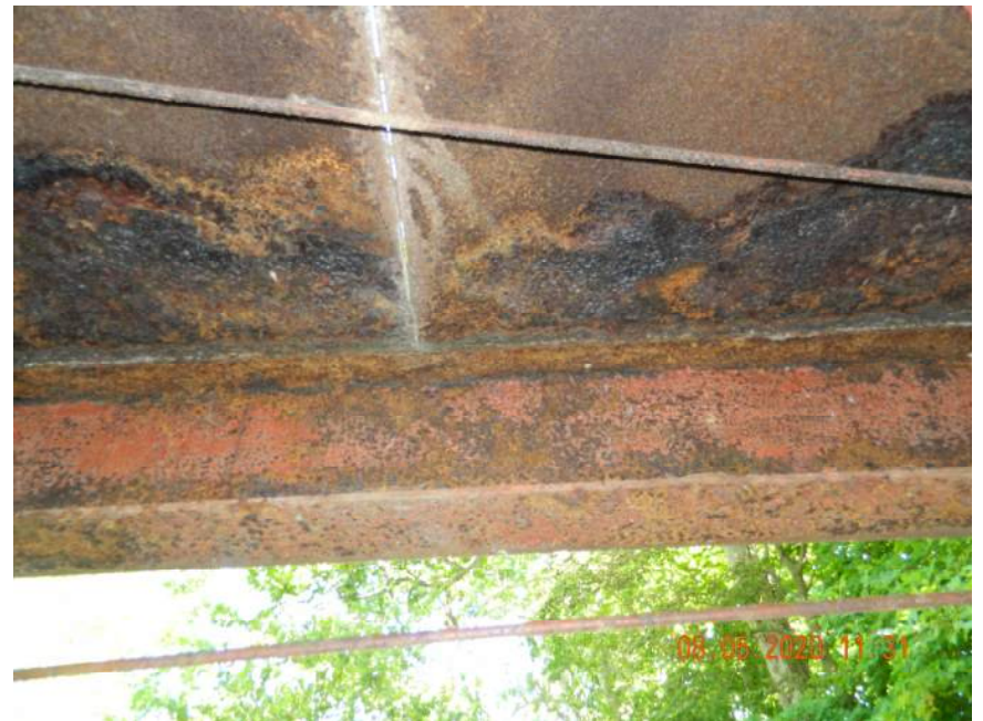
TYPICAL PACK RUST AT STEEL BEAMS & DECK PL
