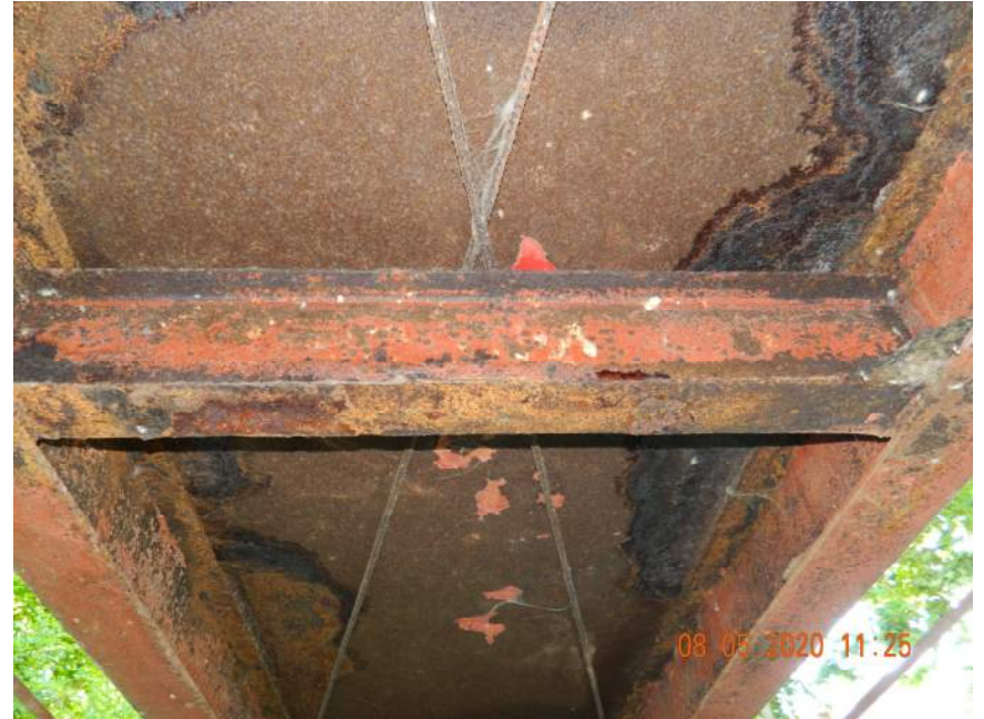
HEAVY RUST IN STEEL DIAPHRAGM
