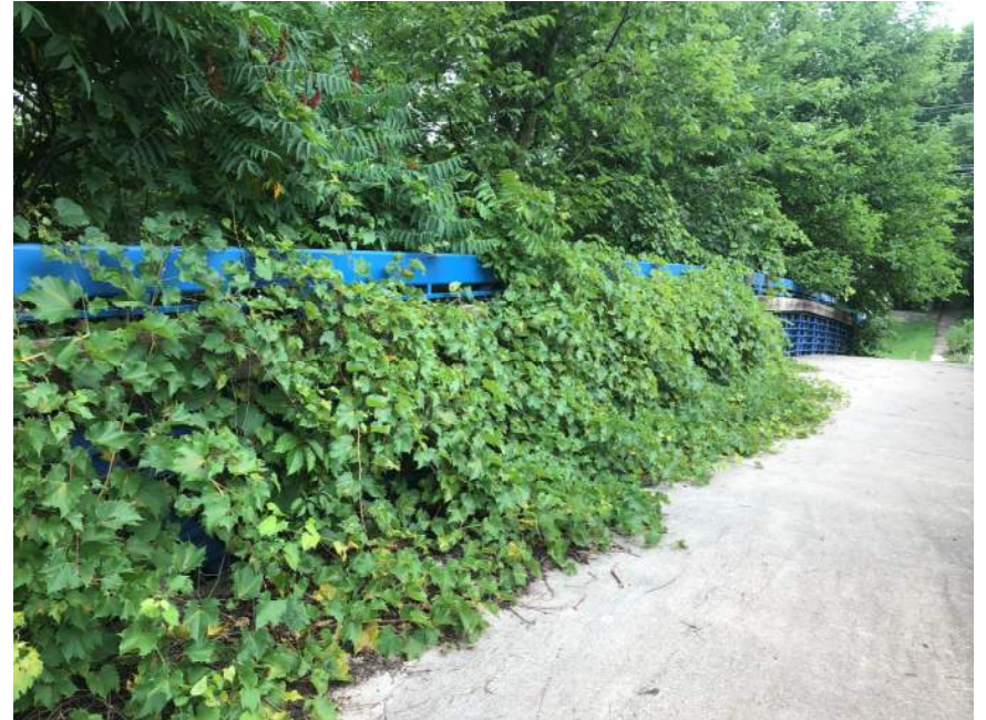
HEAVY VEGETATION ON WEST TRUSS
