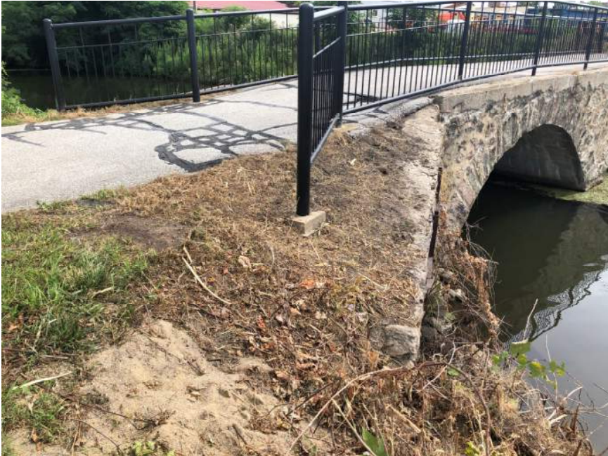
EROSION AT SOUTHWEST WINGWALL
