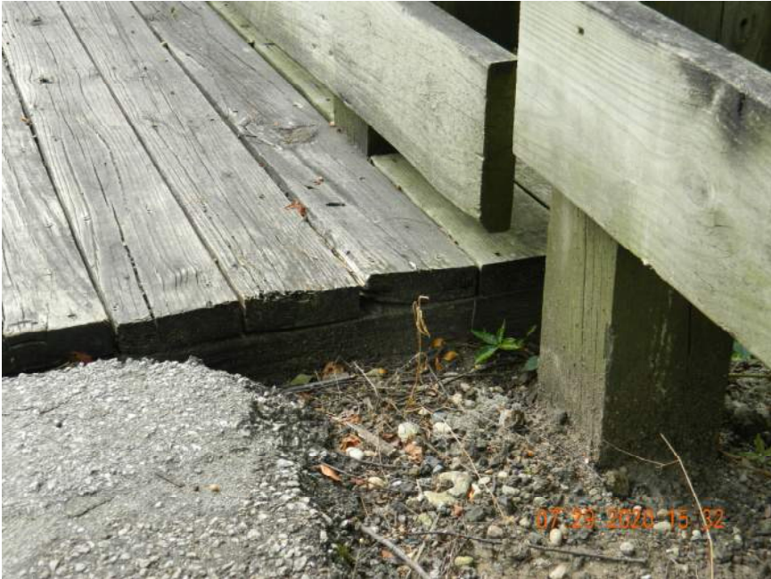
EROSION BEHIND SOUTHWEST CORNER
