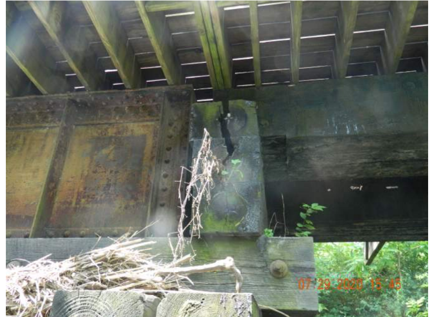
LARGE SPLIT IN TIMBER CAP OF EAST PIER OF MAIN SPAN
