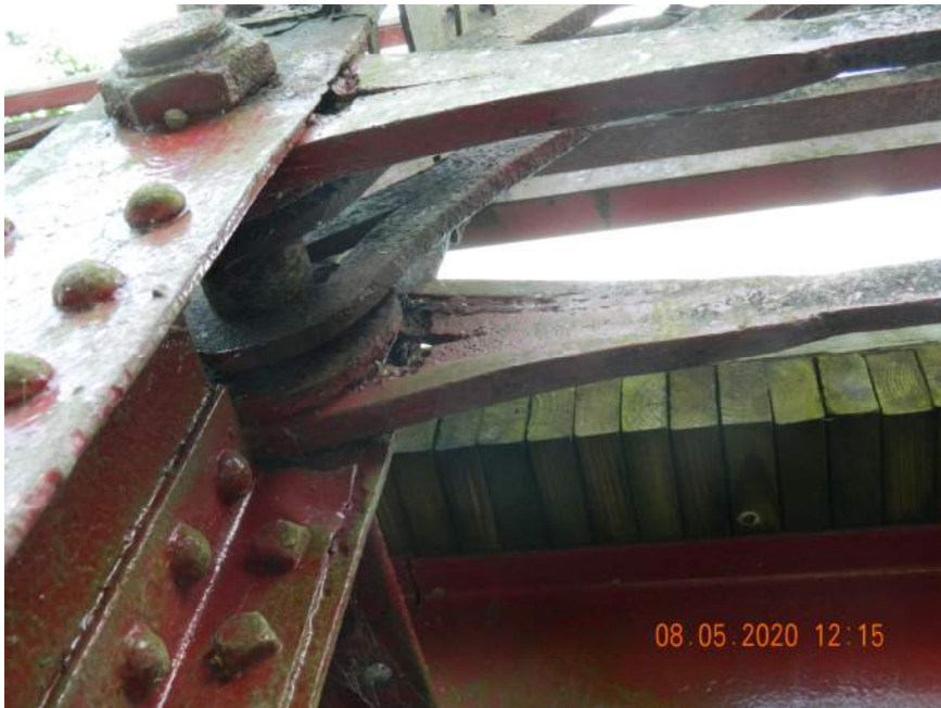
TYP. PACK RUST AND SECTION LOSS AT EYEBARS
