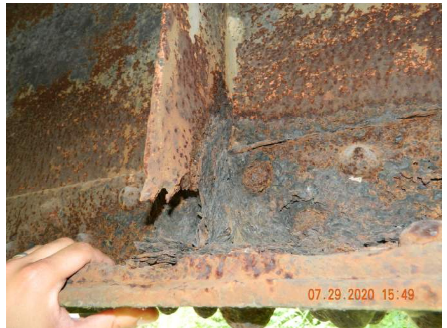
HEAVY PACK RUST AND PITTING AT STEEL STIFFENERS
