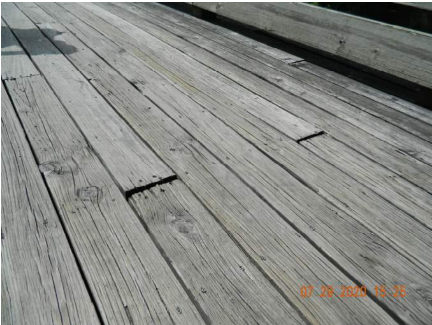
TIMBER DECK BOARDS PRYING UP
