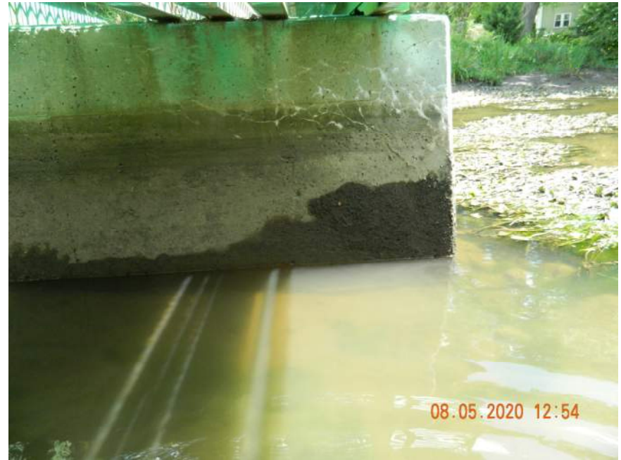
SCOUR DEPRESSION AT SOUTH END OF WEST PIER
