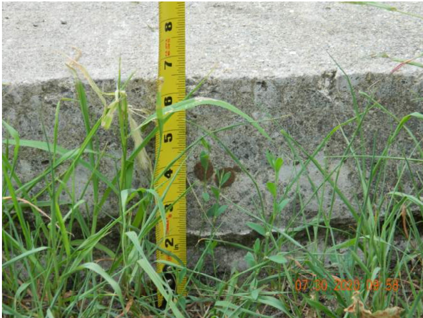
6.5" DROP OFF AT NORTH APPROACH
