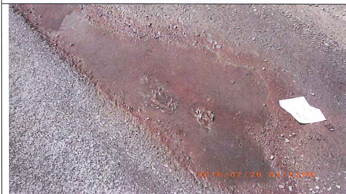
Photo 7 – Another discolor pool of water along internal access road.
