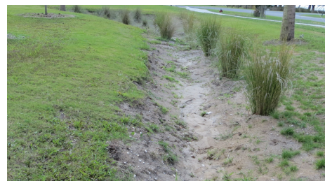
8 INLET EROSION (GRASS CHANNEL)
