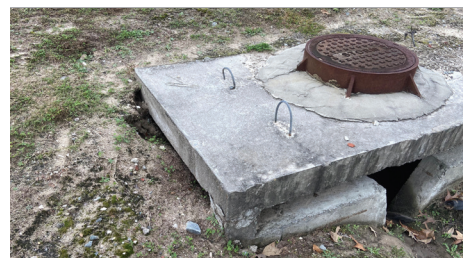
19 OUTLET STRUCTURE EROSION
