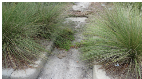
5 INLET STRUCTURE DEBRIS & SEDIMENT
