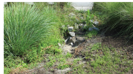
8 INLET EROSION (ROCK PLUNGE POOL)
