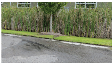
11 EXCESSIVE PONDING (CATTAILS & STAINING)
